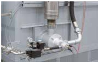
Gas burner positioned along the furnace side
